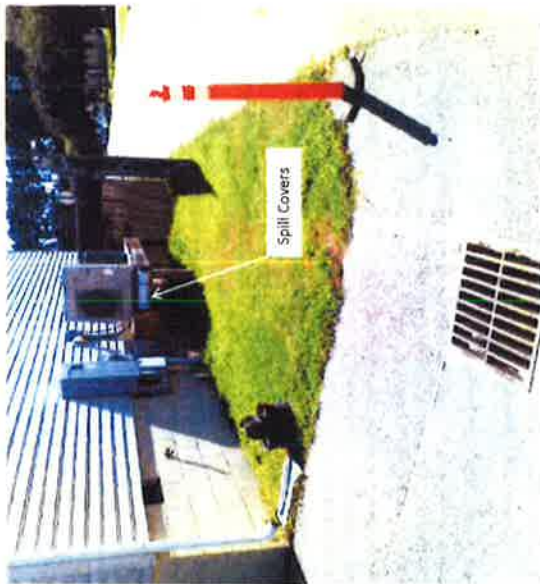
Figure 7 Drop Inlet Spill Covers
