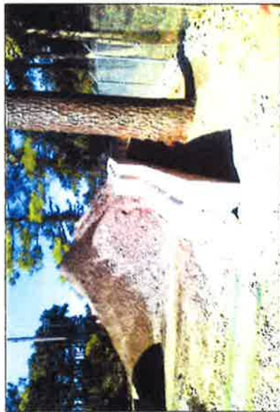
Figure 9 Rock Check Dam Against Perimeter Fence
